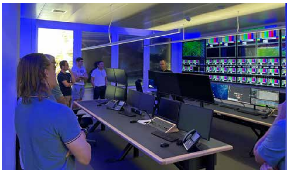
Einblick in den Master Control Raum. Foto: Patrik Sanader, NEP Switzerland
